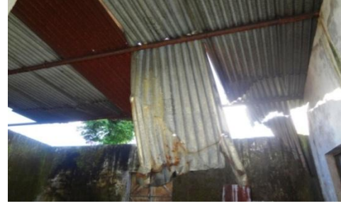
Abandoned Indragarh 33 no. AWC under Tapang ICDS Project, Cachar (21.07.2014)
