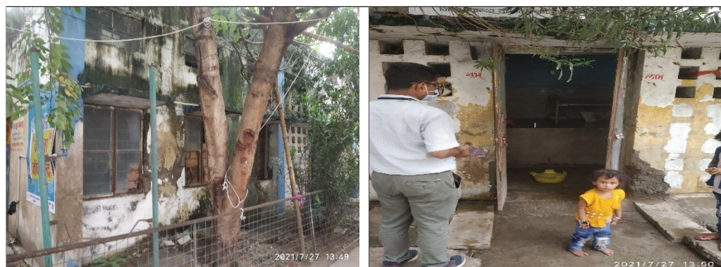
Kitchen at DH-Jehanabad in a condemned building
